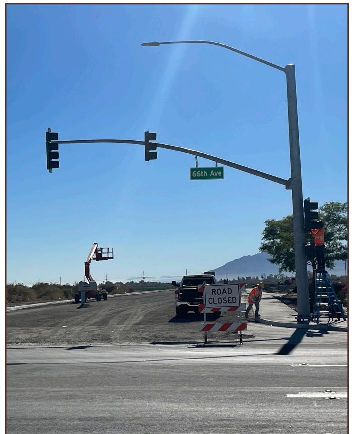
Crews installing the new traffic signal at the new Dale Kiler Road and Avenue 66 Bypass Road intersection. The sidewalk, curb and gutter is complete with paving coming soon. The new road will open early next year.
